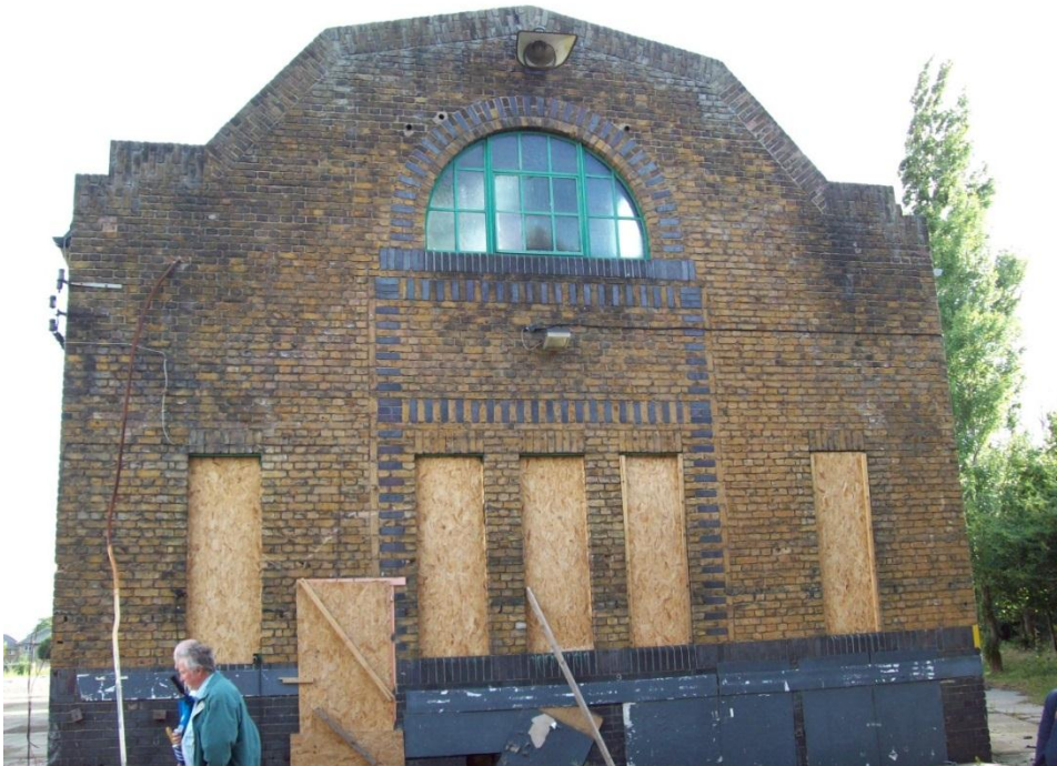
Fig. 16 The Power House
