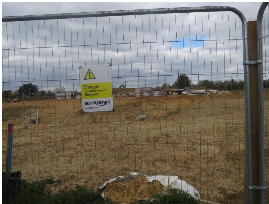
Figure 9: View from the footpath to the rear of Threshelfords into the new housing development
