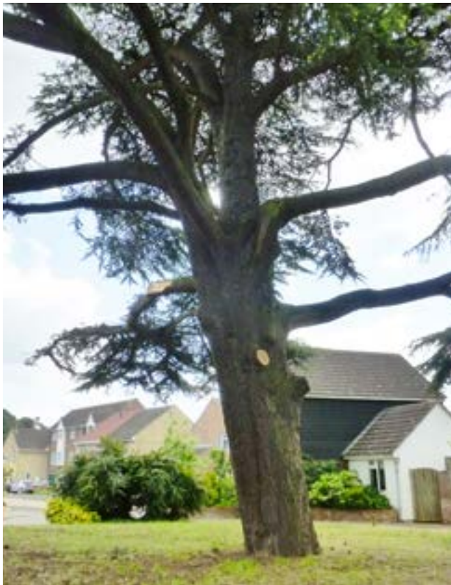
Plate v – b & c Cedar after storm event and trimmed for canopy damage in early June 2015 – tear damage from falling limb evident in second photo.
