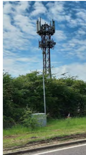
Mobile Mast near The Vineyards
